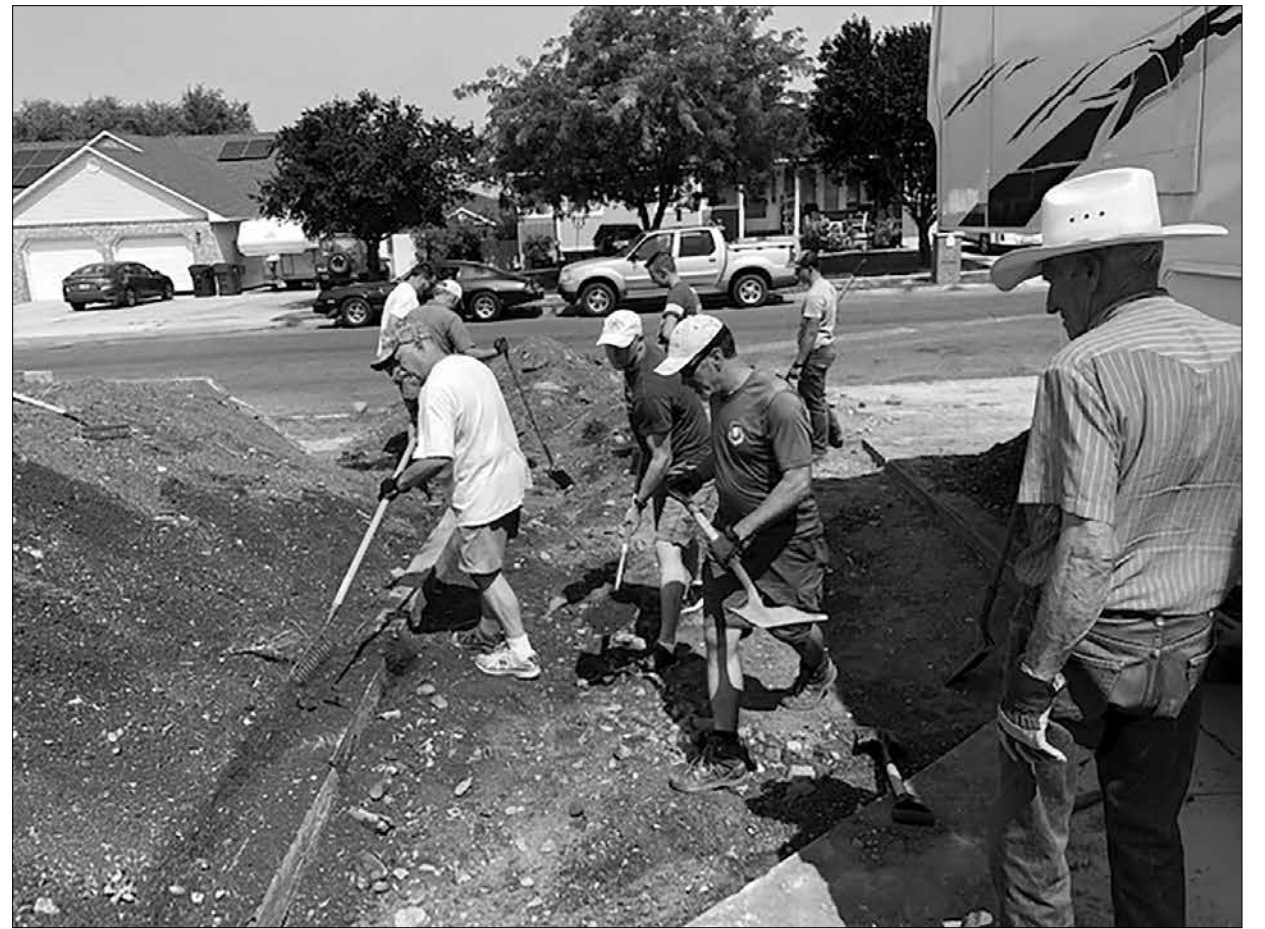
Volunteers work to expand the Bartlow family's driveway to make access easier loading Ellie in and out of their vehicle.
