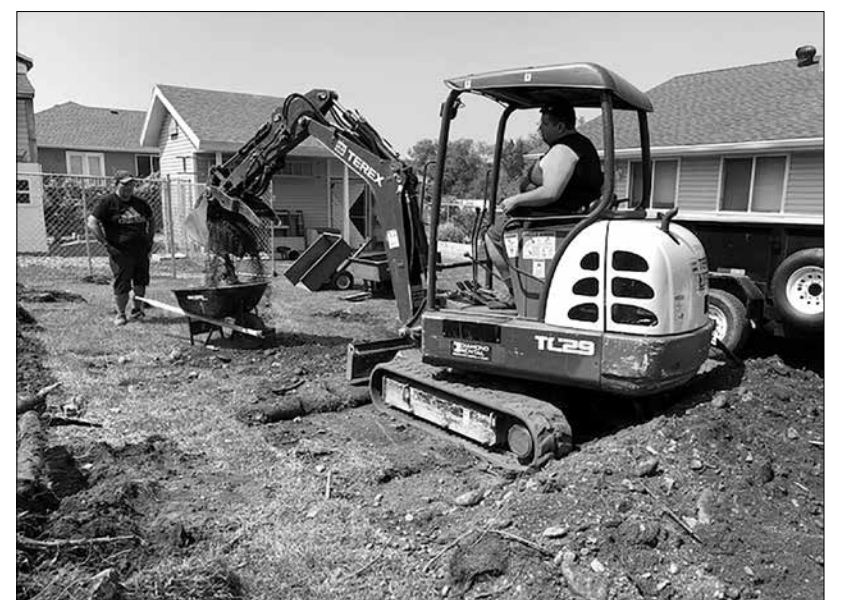
An excavator was used to pull up sod to prepare for a back driveway at the Bartlow home, in order to make transporting Ellie less strenuous.
